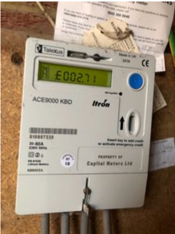
Utility Photo - Provided by inspector
