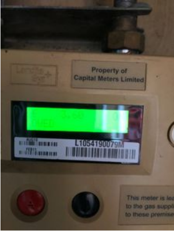
Utility Photo - Provided by inspector
